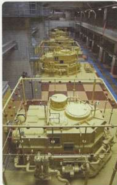
View of pump room
